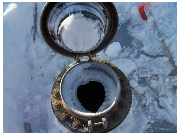
Figure 17: Frost Closure of a Tank Vent (VGH)
